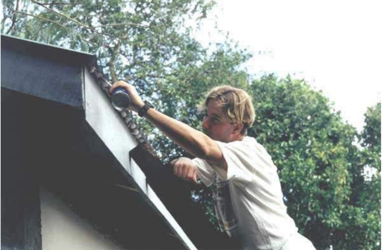
Figure A1:9. The grantee applying expanding foam sealant to the holes created by the metal roof.
